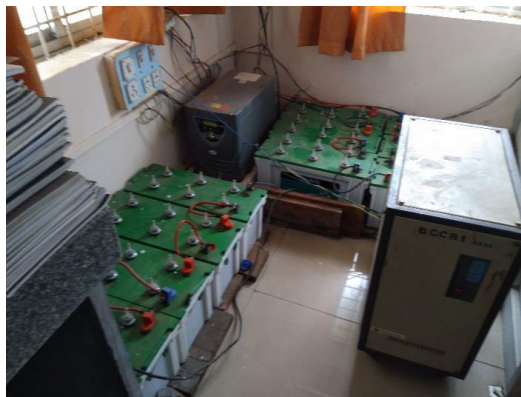
Batteries stacked for disposal
